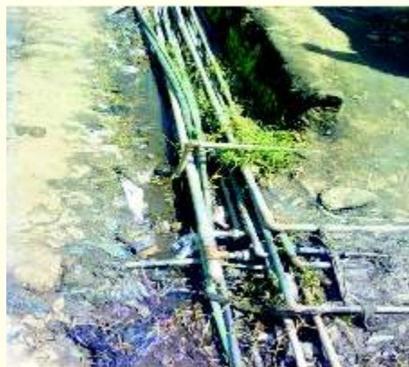
Burst leaking pipes as source of drinking water
